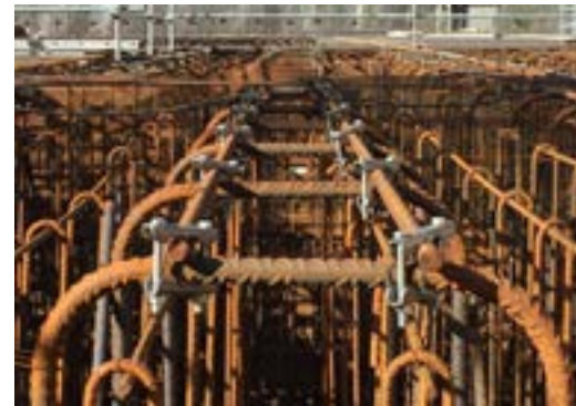
Reco 'CBL' Clamp (as used on Hinkley Point C) – a lifting clamp for connecting 'Cross Bar' perpendicular reinforcement
